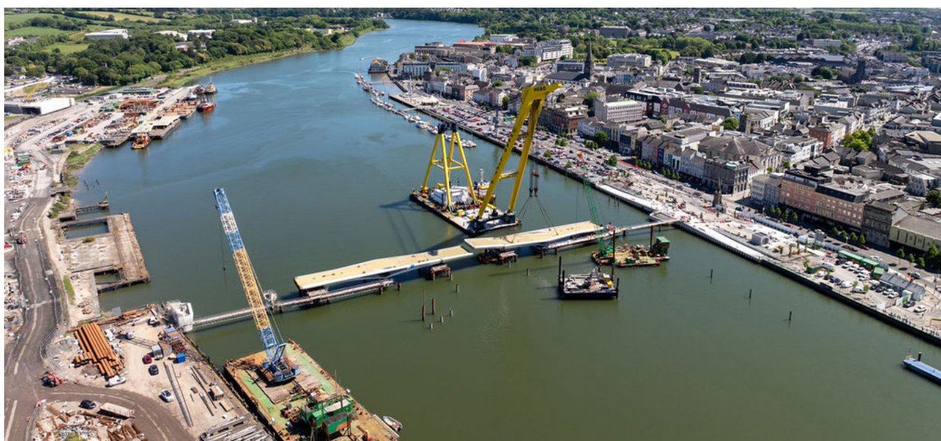
Figure 2: Installation of Sustainable Transport Bridge to North Quays (Source: Waterford City and County Council)
