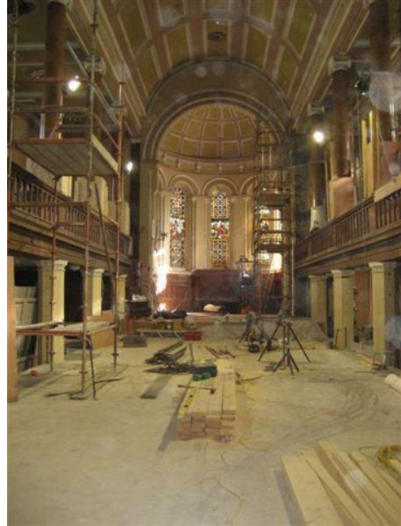
Interior of Christchurch during refurbishment works. Image courtesy of Cork City Council.
